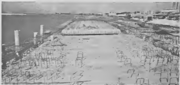
Section of new pier on HDS site, looking west. Parti di e pier nobo ariba tereno di HDS, mirando west.
